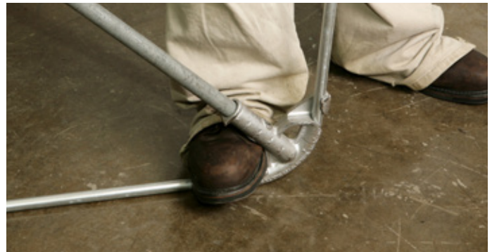
The NEC requires metal enclosed wiring if you use OBC AFCIs on the home run.
